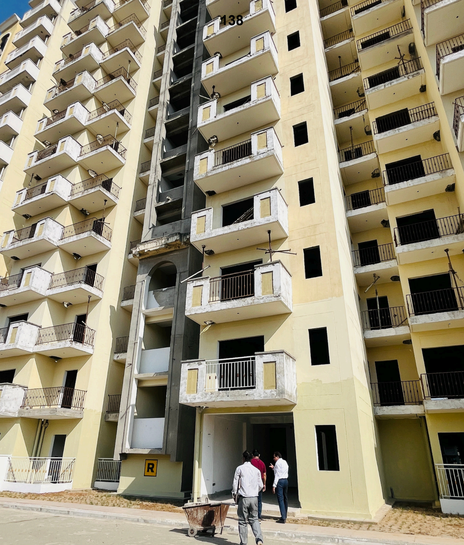
Photo of Tower R as on 4 th November In the presence of IRP Dr. Lekhraj Bajaj & Monitoring Committee President Mr Gaurav Khanna
