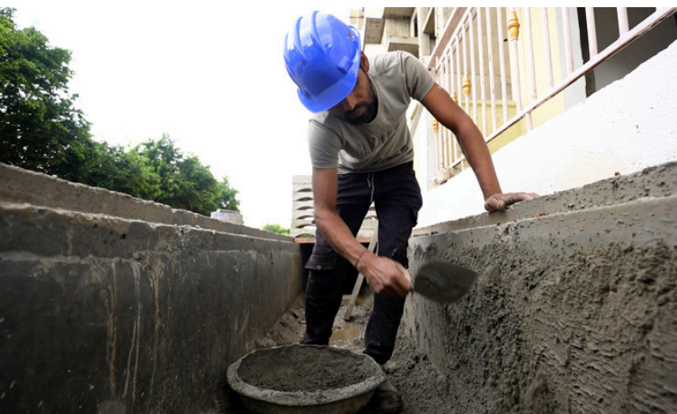
water proof plaster inside the drain
