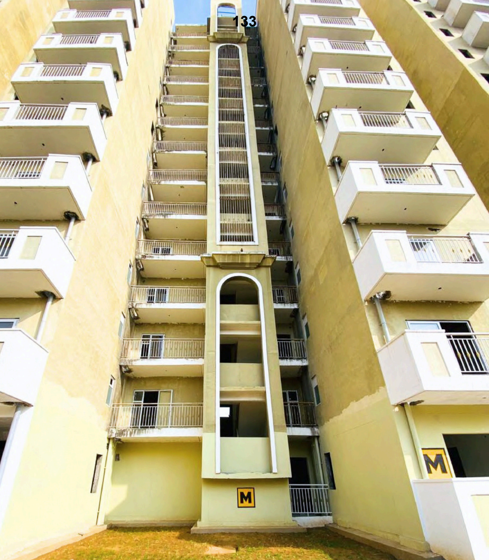
Photo of Tower M as on 4 th Nov 2025 during the visit of IRP Dr. Lekhraj Bajaj & Monitoring Committee President Mr Gaurav Khanna
